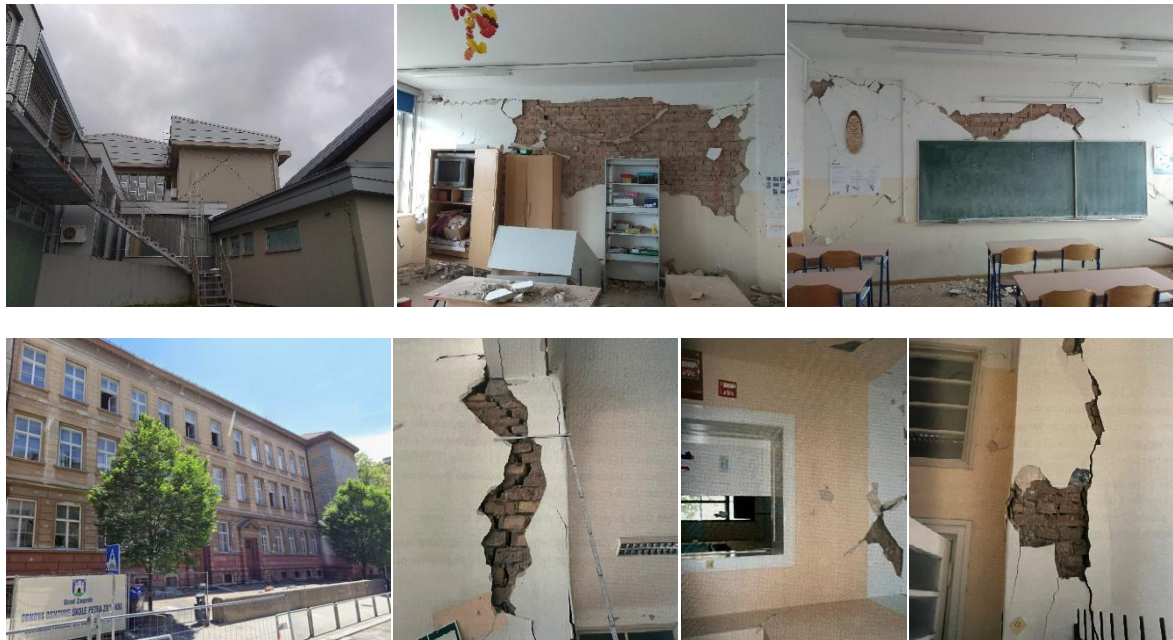
Figure 7- Damage to elementary school buildings: Vugrovec-Kašina (top) [27] and Petar Zrinski [28] (bottom)
