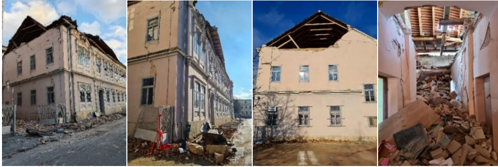
Figure 9- Damage to Petrinja Elementary School [27]
